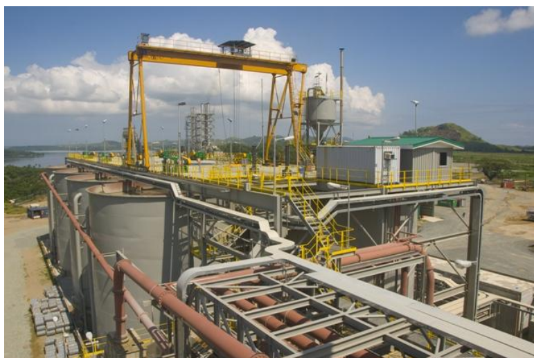
Masbate Gold Project – CIL Tanks
